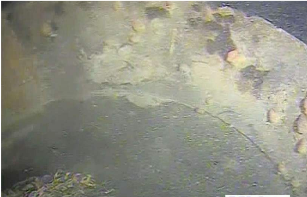
Figure 9 – Existing Tank Interior (2018) Showing Corrosion
