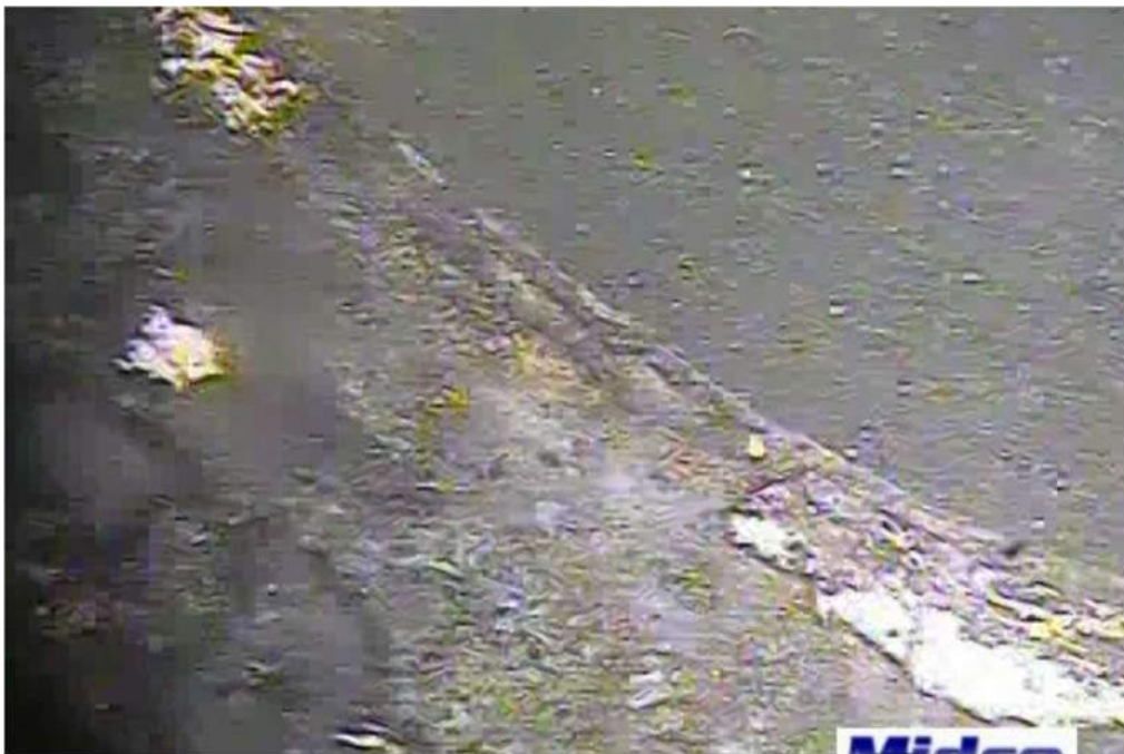
Figure 10 – Existing Tank Interior (2018) Showing Corrosion
