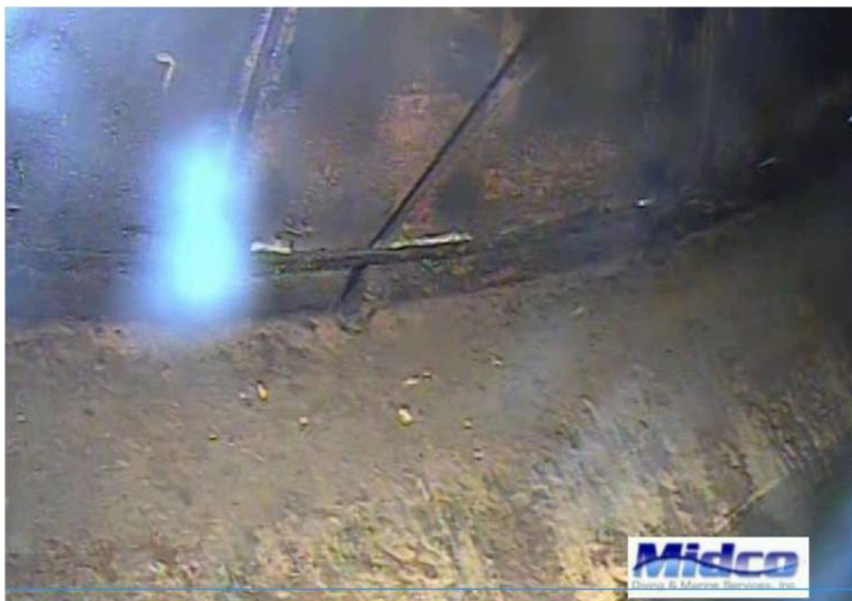
Figure 8 – Existing Tank Interior (2018) Showing Corrosion and Daylighting Above Waterline
