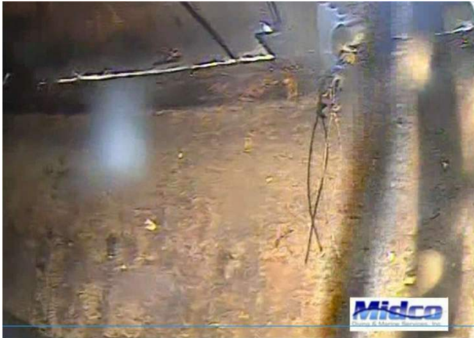
Figure 11 – Existing Tank Interior (2018) Showing Corrosion and Daylighting Above Waterline
