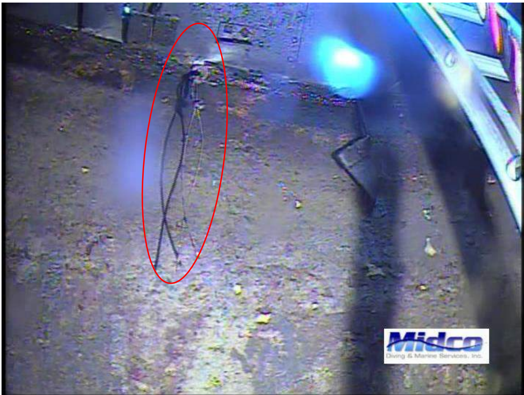
Disconnected Wires Noted
