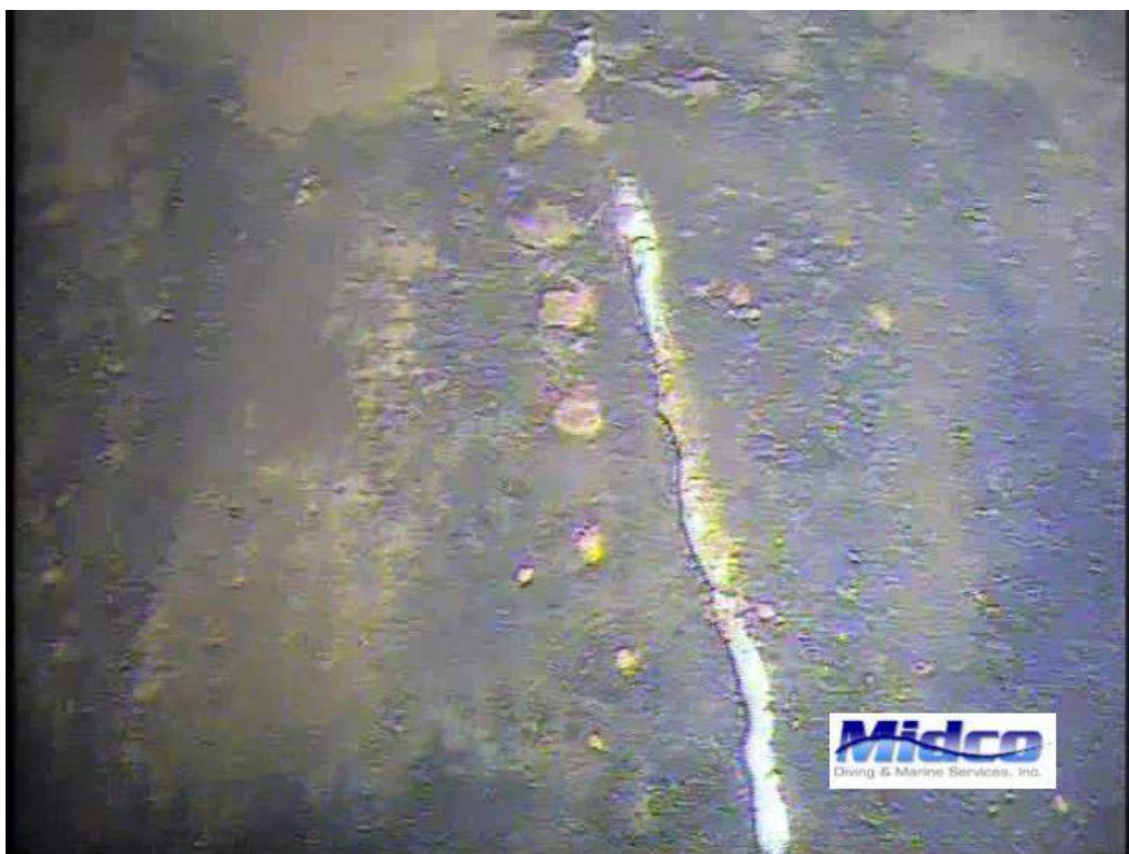
Previous Epoxy Repairs Noted on Floor
