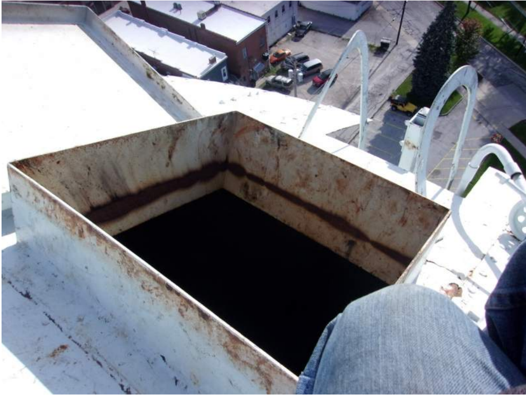
Access Hatch – No Weather Stripping Noted
