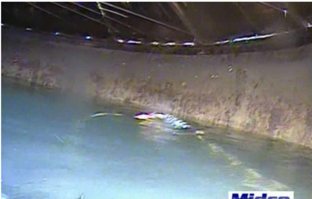
Figure 12 – Existing Tank Interior (2018) Showing Corrosion and Daylighting Above Waterline
