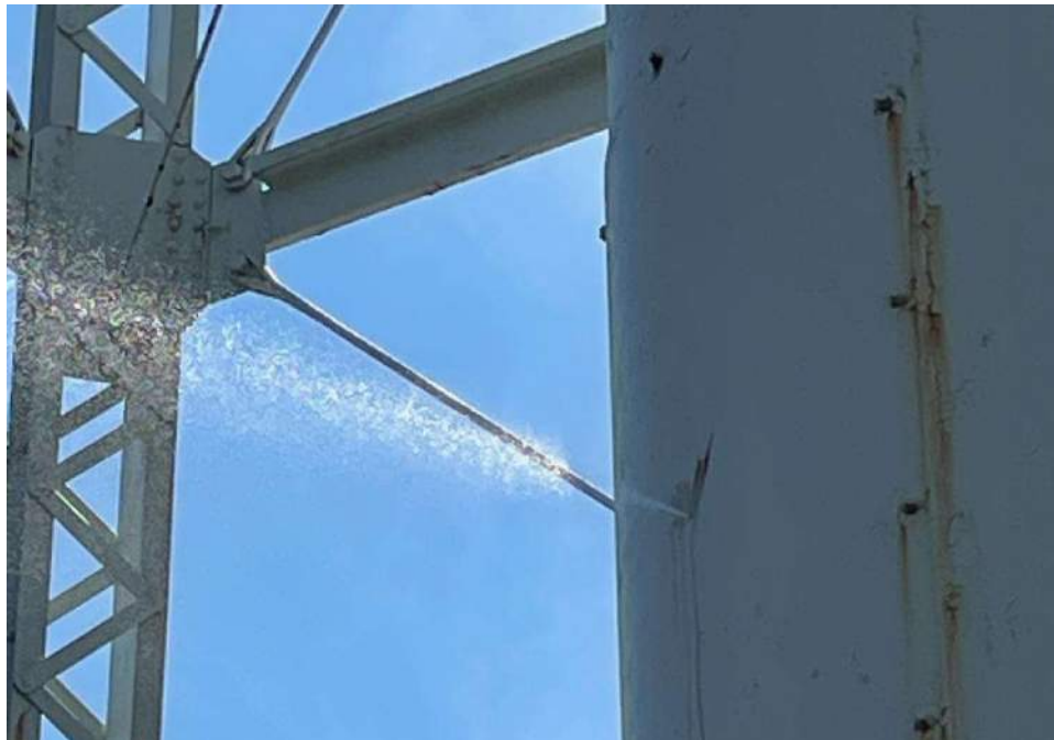
Figure 2 – Major Leak in Riser Pipe of Existing Pemberville Water Tower on August 23, 2022
