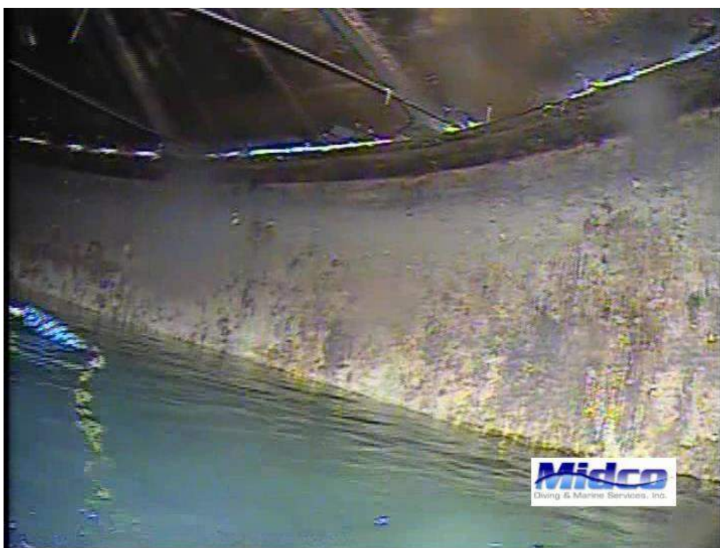
Wall to Roof Seam – Daylighting Noted
