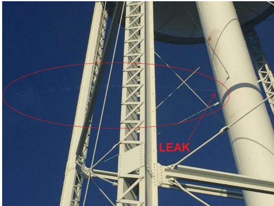
Figure 5 – 2016 Major Leak in Riser Pipe of Existing Pemberville Water Tower
