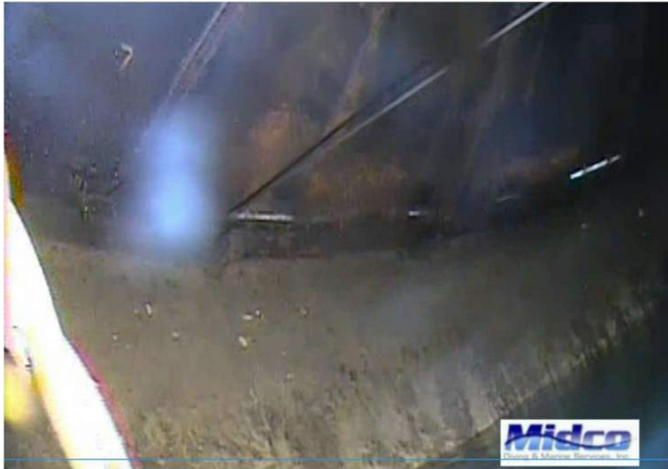
Figure 13 – Existing Tank Interior (2018) Showing Corrosion and Daylighting Above Waterline
