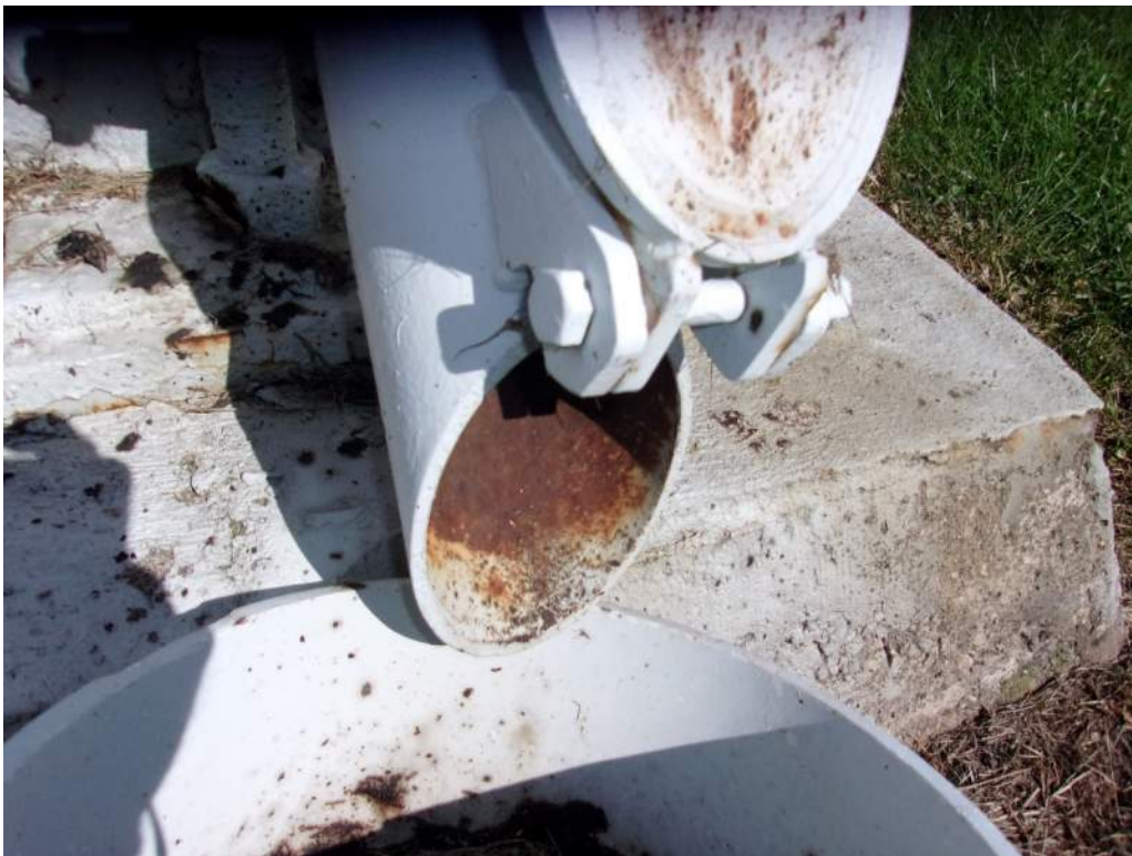
Overflow Plumbing – No Screen Noted
