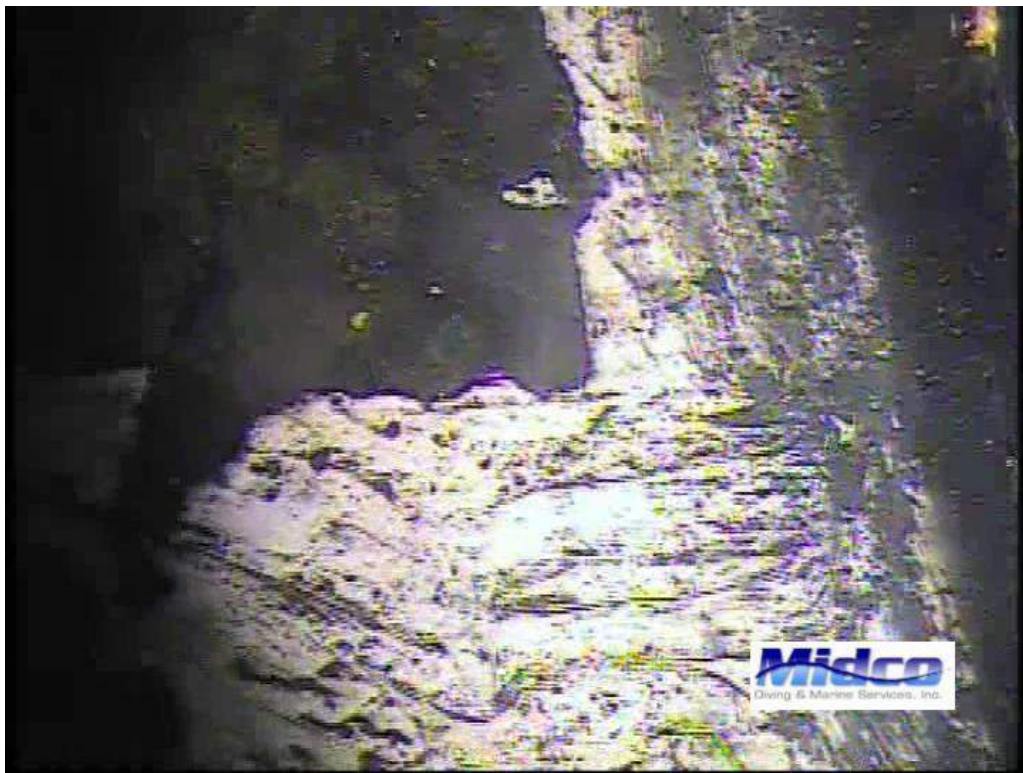
Previous Epoxy Repairs Noted on Floor
