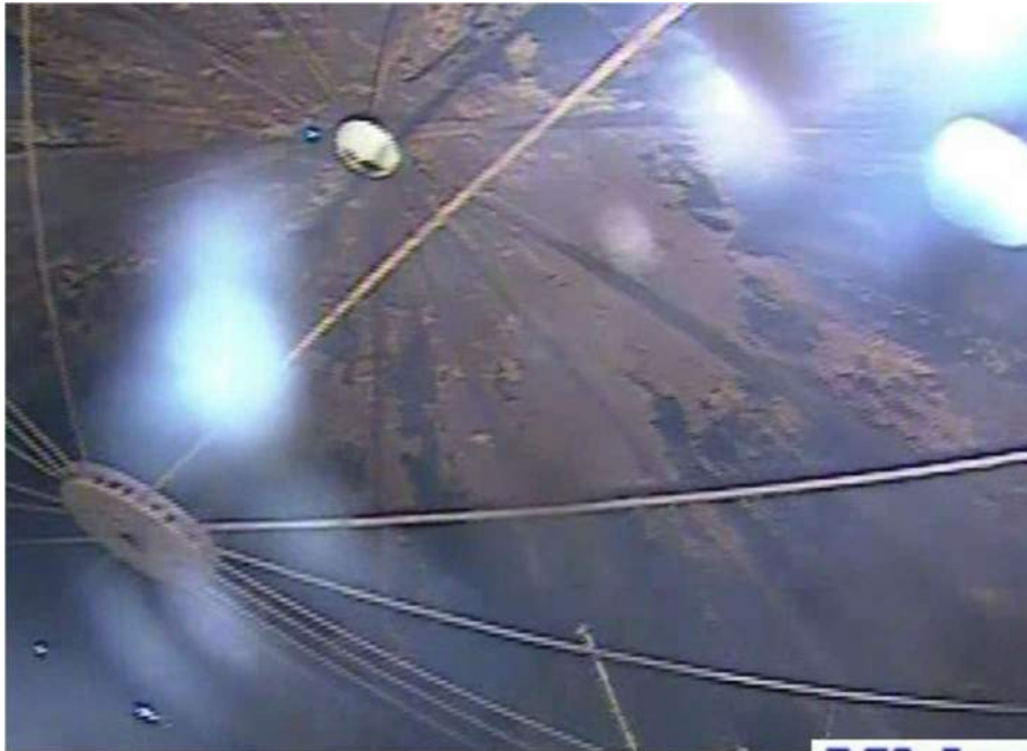
Figure 7 – Existing Tank Roof (2018) Showing Corrosion and Daylighting Above Waterline
