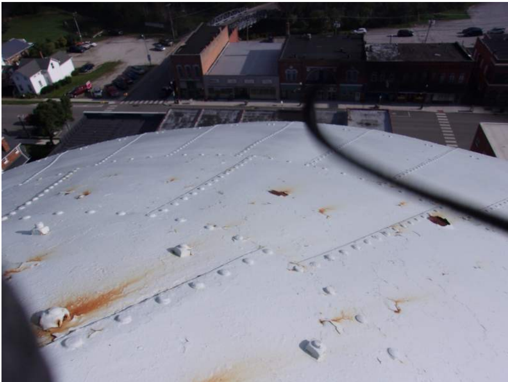
Reservoir Roof – Coating Failure with Corrosion Noted
