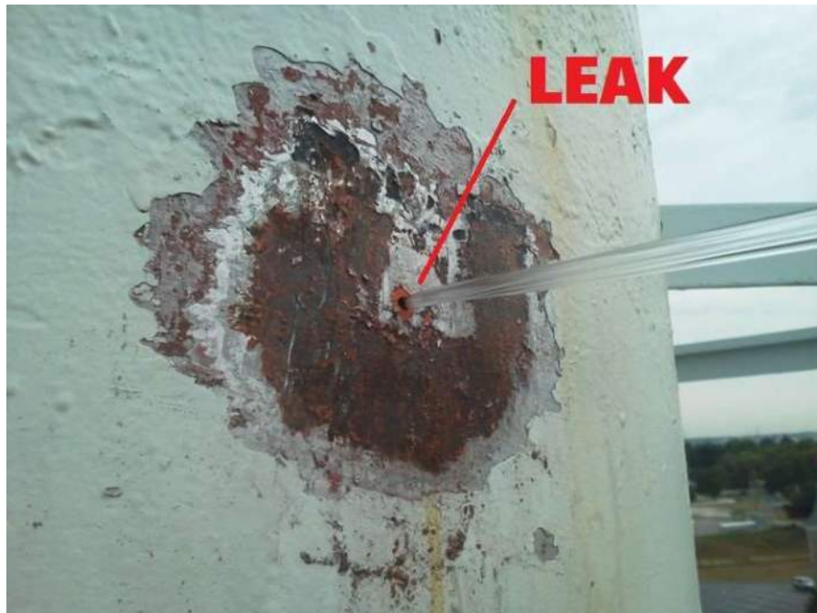
Figure 4 – 2016 Major Leak in Riser Pipe of Existing Pemberville Water Tower
