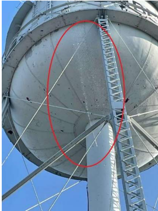
Figure 3 – Major Leak in Riser Pipe of Existing Pemberville Water Tower on August 25, 2022
