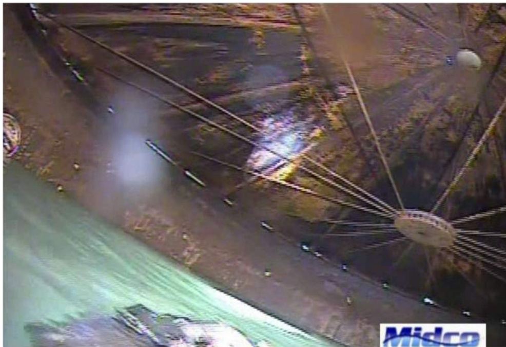
Figure 6 – Existing Tank Interior (2018) Showing Corrosion and Daylighting Above Waterline
