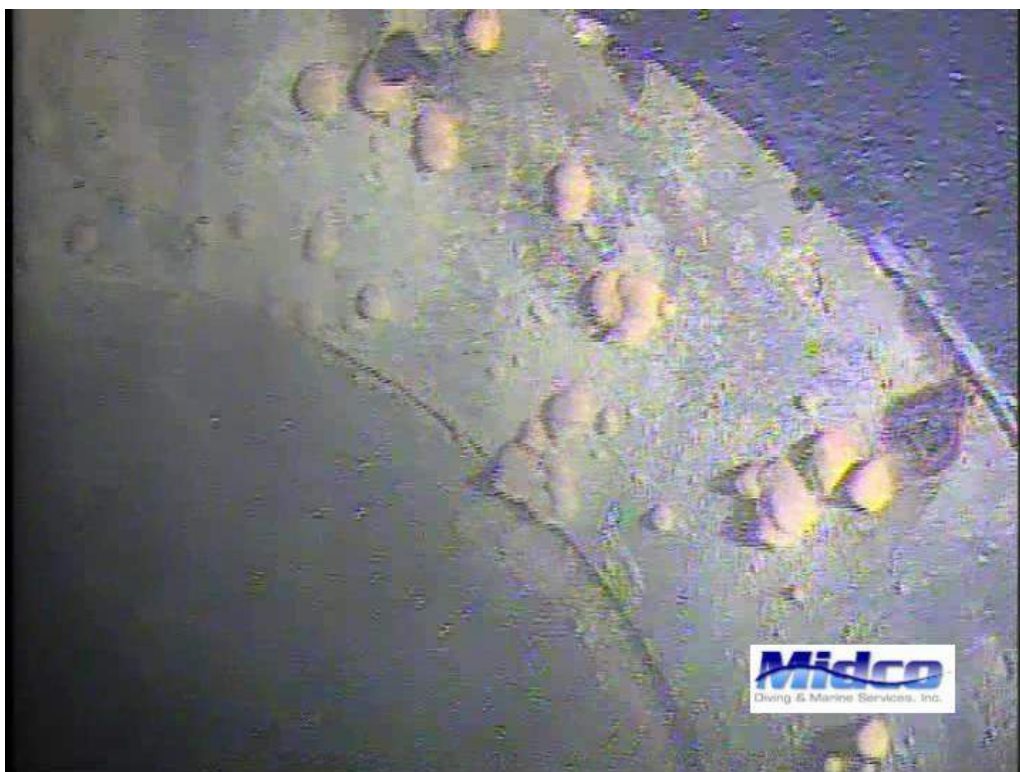
Common Inlet/Outlet – Coating Failure with Corrosion Noted
