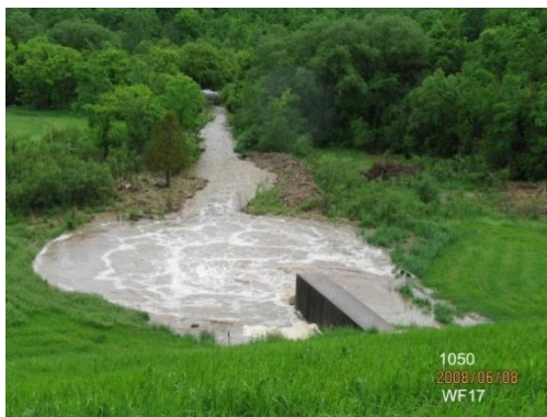
West Fork 17 Stilling Basin Damage – June 2008
