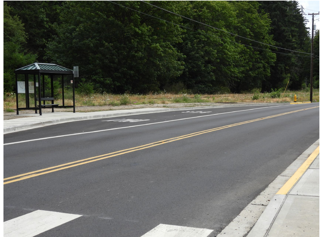
Western Gateway – New paving at Pacific Court and new bus pullout and shelter
