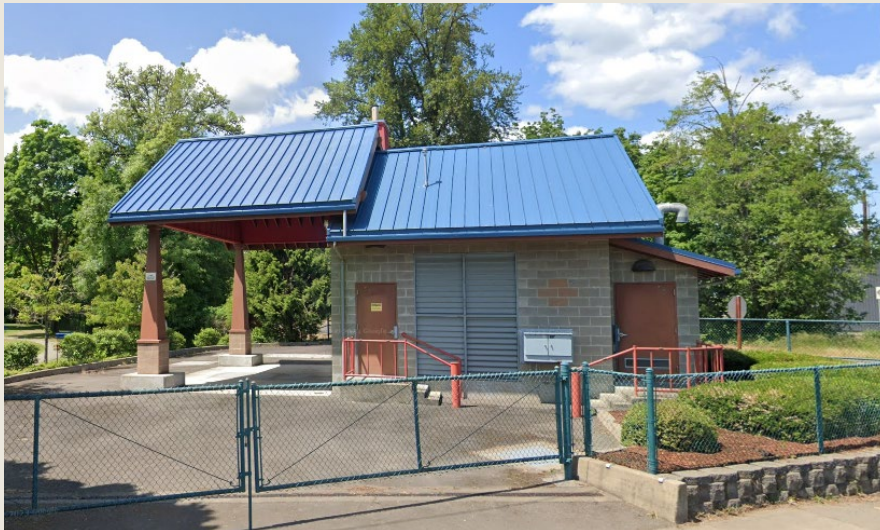
Kneeland Lift Station
