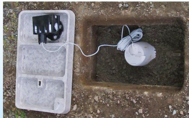
Typical Meter & Transmitter Installation
