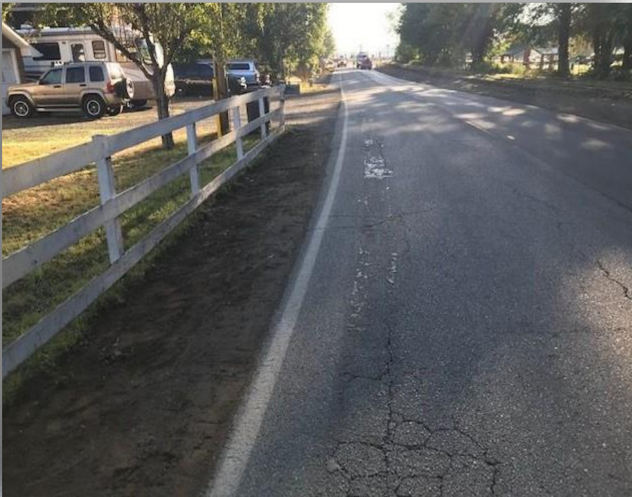
Park Street before 2021 overlay
