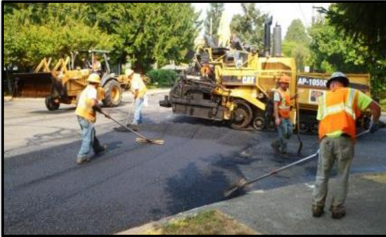
Pavement overlay: Thin lift overlays, thickness of 1-inch. Standard overlays are about 2-3 inches of asphalt. Park Street 2021.
