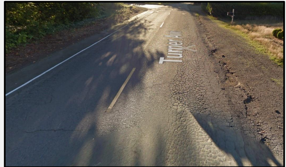
Full Depth Replacement: The existing pavement section is pulverized and reused or replaced. Very expensive when compared to street overlays. Turner Avenue 2018.
