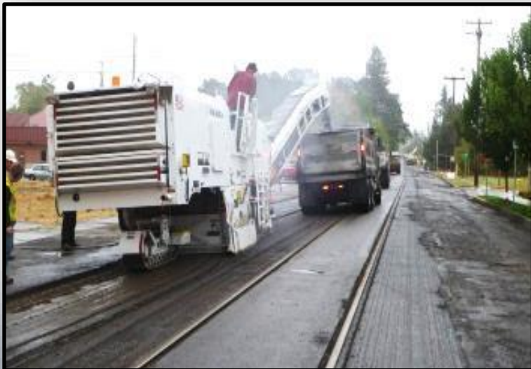
Pavement grinding and inlay: Used on severely distressed pavement that has an adequate baserock section, or when existing surface elevations need to be maintained.
