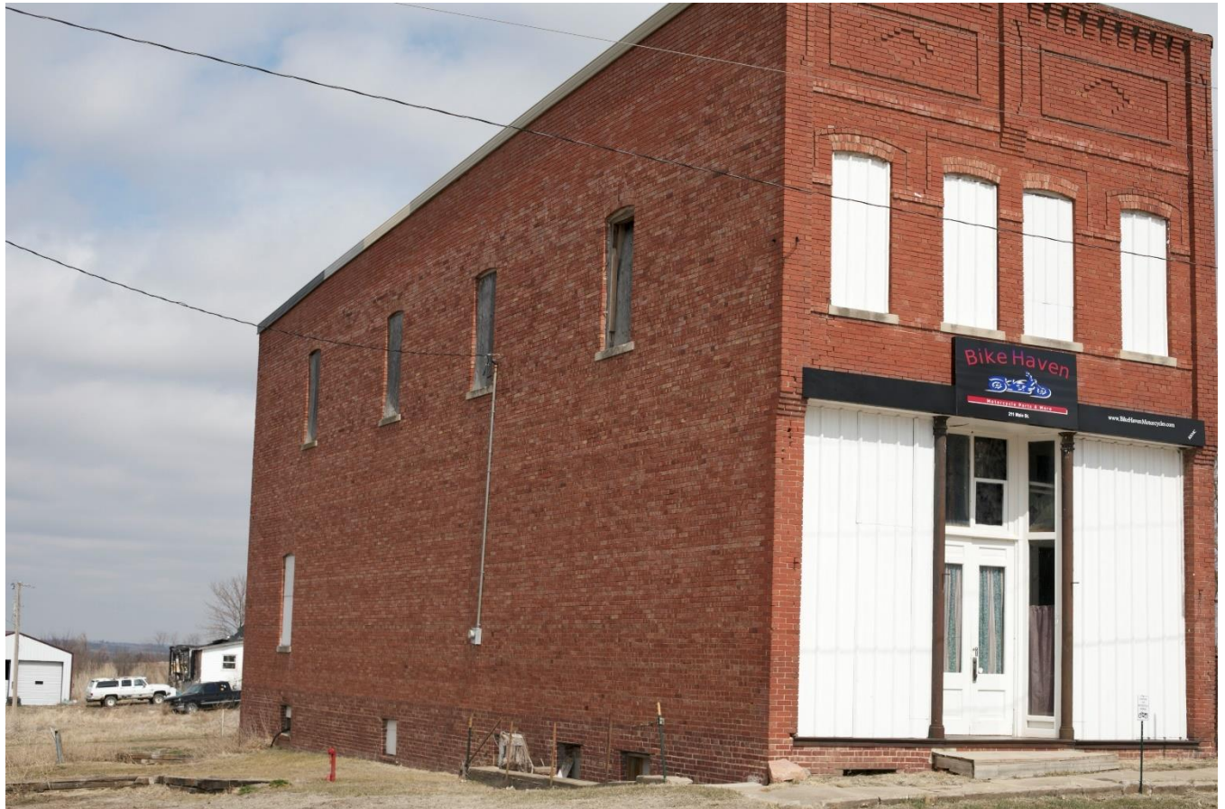
West and south sides of the building, looking northeast. Photo: Kim Scharfenkamp, March 2023.
