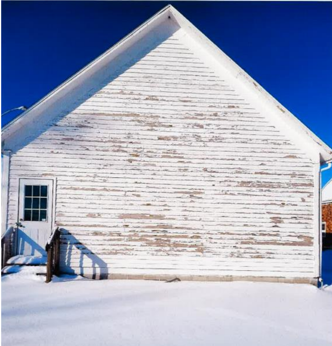
South side of the school museum, looking north. Photo Source: Marlene Tull, January 2023
