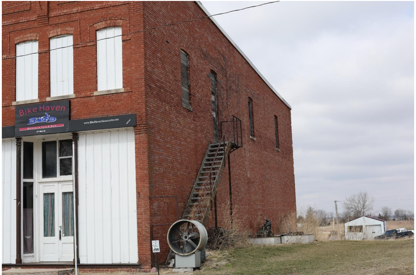
East and south sides of the building, looking northwest. Photo: Kim Scharfenkamp, March 2023.
