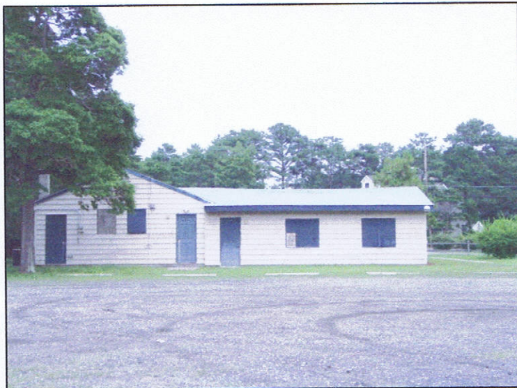
Country Lakes Recreation Center is the main office for the Recreation Department. The building needs some minor renovations such as exterior painting, new doors and new windows.
