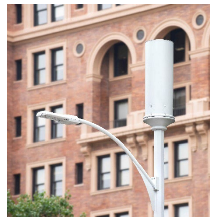
(Above) Installation of 5G Service: High-speed internet refers to internet connections with download speeds of 25 Mbps or faster
