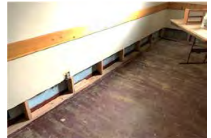
Interior of basement living space has been mitigated for moisture and mold. Note: No active leaks were observed at the time of our assessment.
