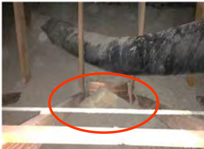
Displaced insulation and visible light from within Parish Center below.
