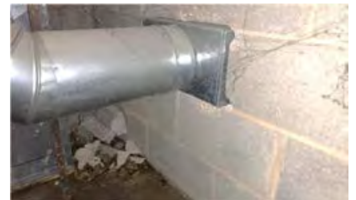
HVAC duct through foundation wall on south wall of mechanical room. No active leaks were observed.
