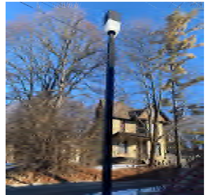
Exterior Light Pole
