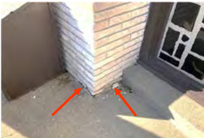
Small amount of deteriorated masonry at the base of the north side of the front Church entrance.
