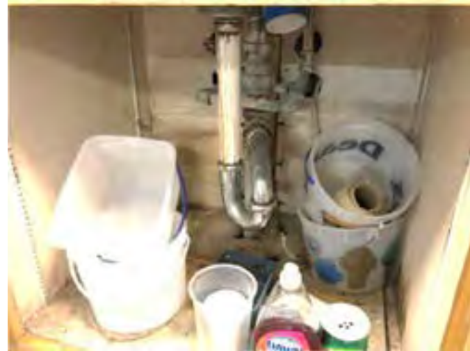
One leak appears to be plumbing related in the basement kitchen.
