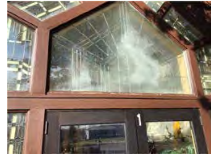
Wood and stained-glass windows show excessive evidence of condensation.
