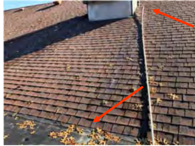
Condensate drain extension from HVAC unit drains onto lower, EPDM roof system
