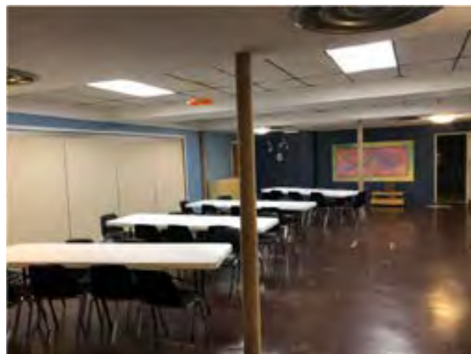
No leaks were observed in the large basement classroom.
