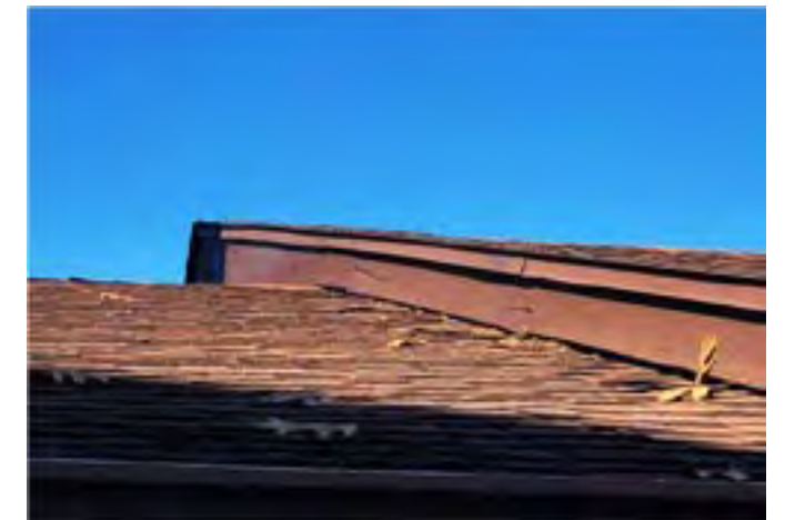
Deteriorated roof rake edge board observed above Narthex area.
