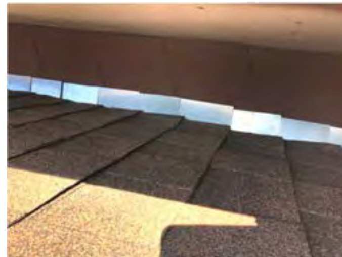
Step flashing under garage addition rake edge overhang. There is no counter-flashing installed over the step flashings.
