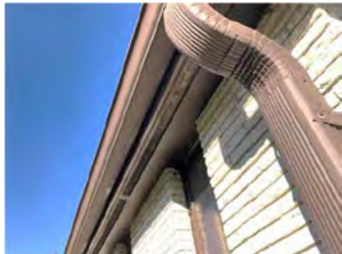
Soffits on south side of Church are also filled with debris from between the rafter spaces.
