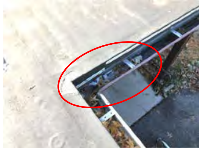
Poor termination bar installation at gutter roof edge.
