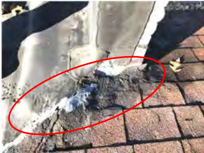
Steep slope roof-to-wall and low-slope to steep slope roof transition with several applications of roof mastic. This is most likely a source for moisture infiltration.
