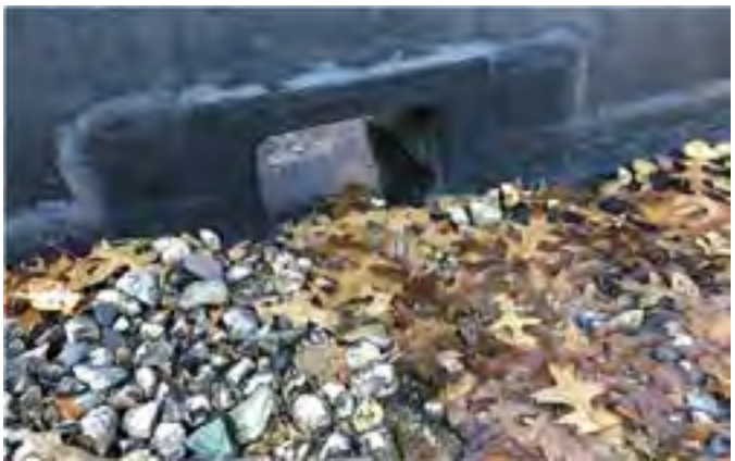
Leaves and debris in through-wall scupper.
