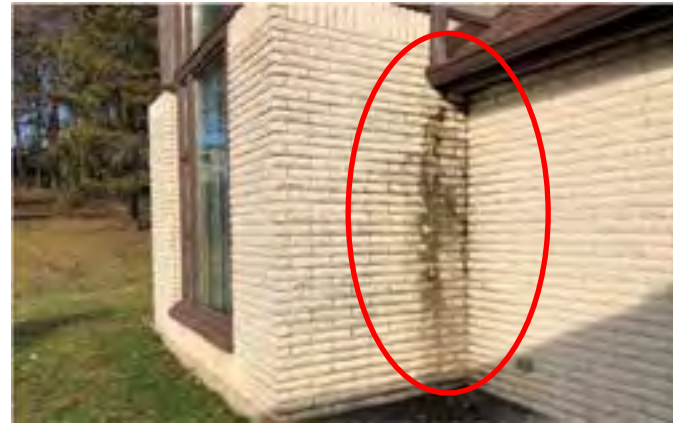
Masonry wall requires cleaning.
