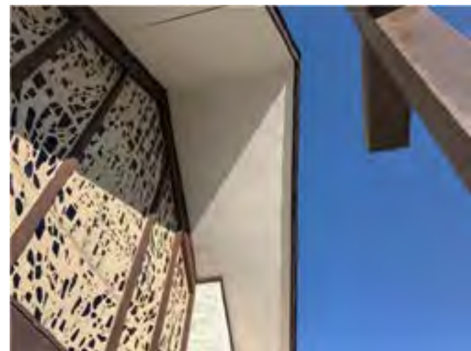
Soffit panels appear to be old and beginning to warp and become dislodged.
