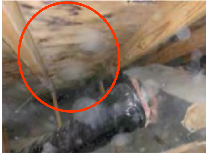
Evidence of moisture staining next to HVAC unit ductwork.
