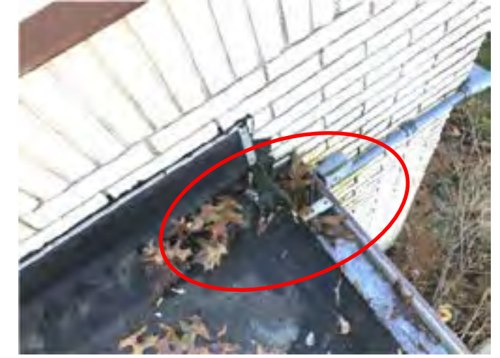
Roof-to-wall/gutter transition. No counter-flashing or through-wall flashing observed.
