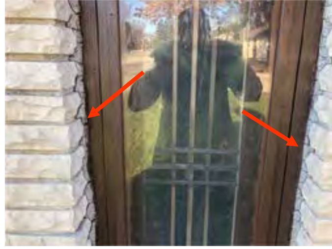
Windows on exterior of the Church Note: Perimeter sealant is in a failed condition.
