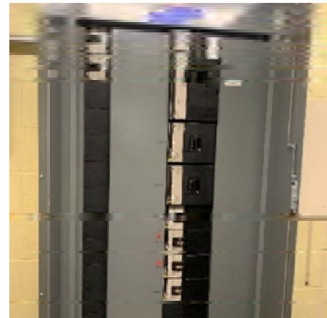
Main Electrical Service Panel
