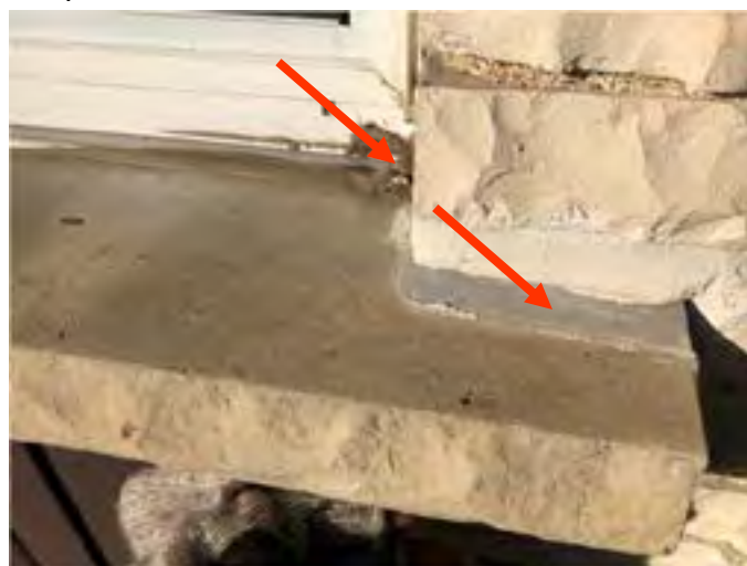
Window sill is loose and sealant has failed.
