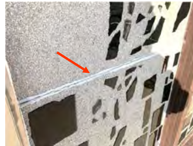
Art Deco panel sealant is in a failed condition.
