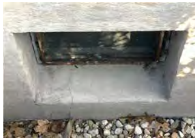
Small shrinkage cracks observed at several light well windows. These do not appear to be structurally compromised.
