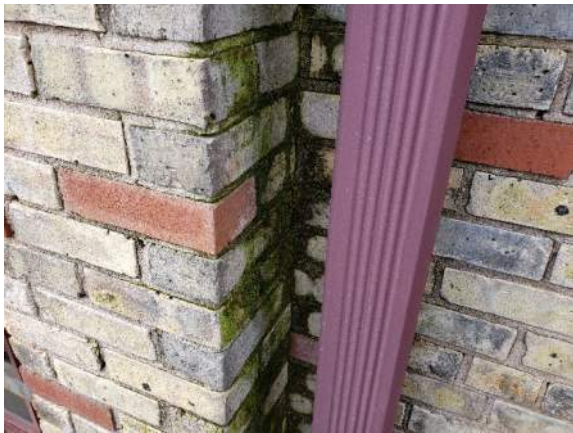
Photo 15- Suspect Biological Growth
