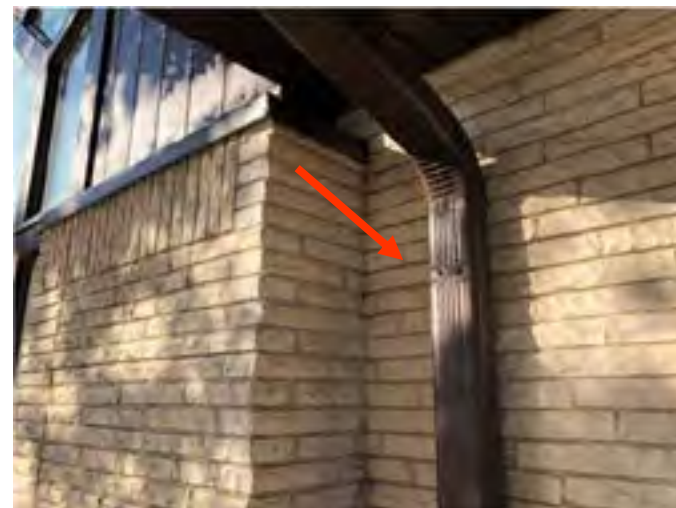
Mortar joint is cracked where masonry steps out.
