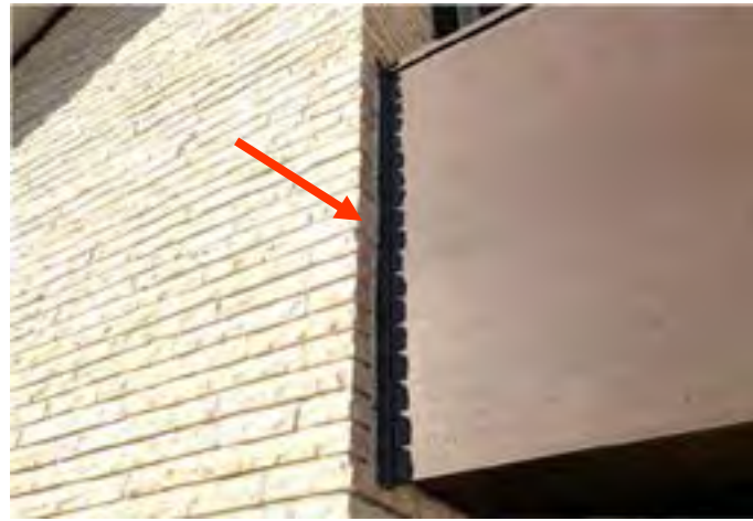
Sealant joint at the masonry to wood panel transition is in a failed condition.
