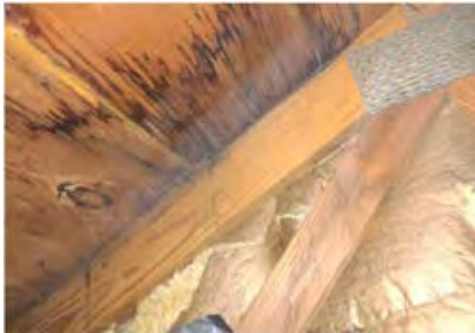
Moisture staining below side of HVAC ductwork/unit curb.
