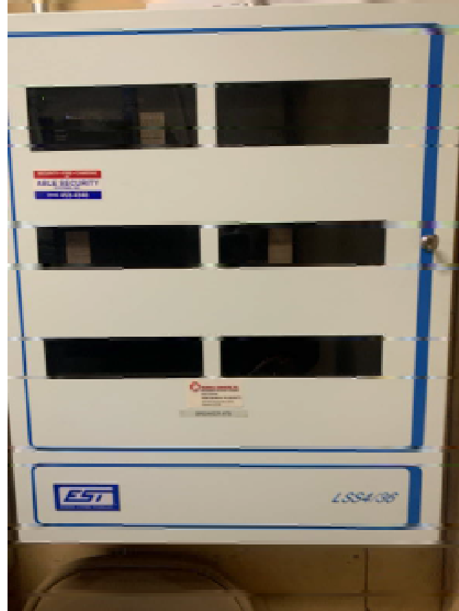
Fire Alarm Control Panel
