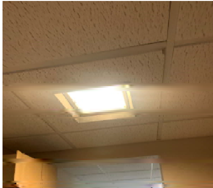
Old Incandescent light fixture
