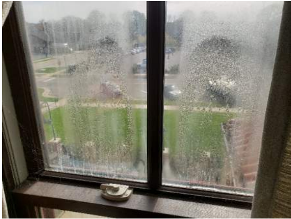
Photo 12 -Broken Window Gasket
