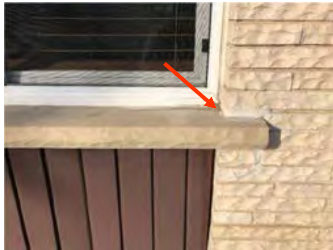
Displaced stone sill.
