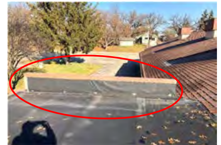
Parapet wall at north end of fully adhered EPDM roof system. Membrane is loose.
