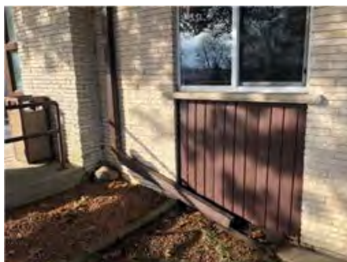
Downspout directs water against metal panel siding.
