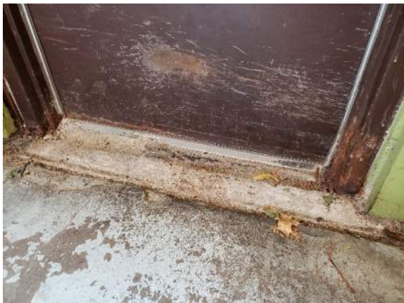
Photo 10 -Door and Frame Corroding
