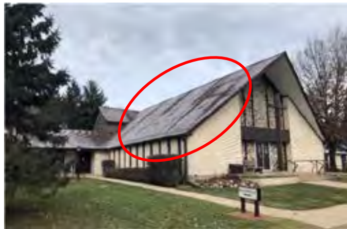
Southwest elevation of Church. Hot spots observed through the frost on southeast slope of Church
