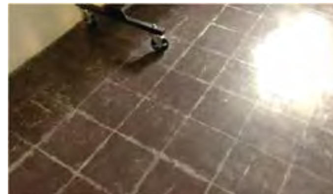
Possible previous moisture observed coming through floor tile seams in stairwell.
