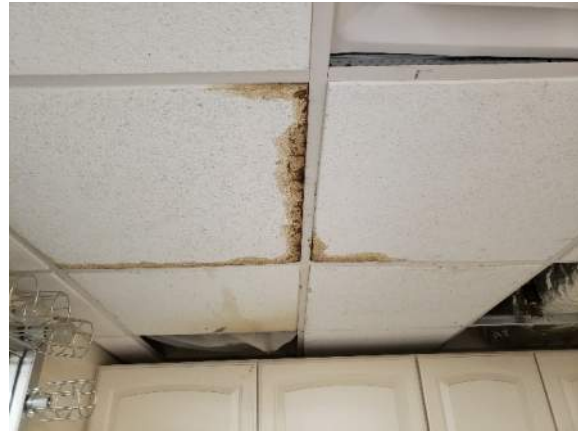
Photo 13- Stained Ceiling Tile
