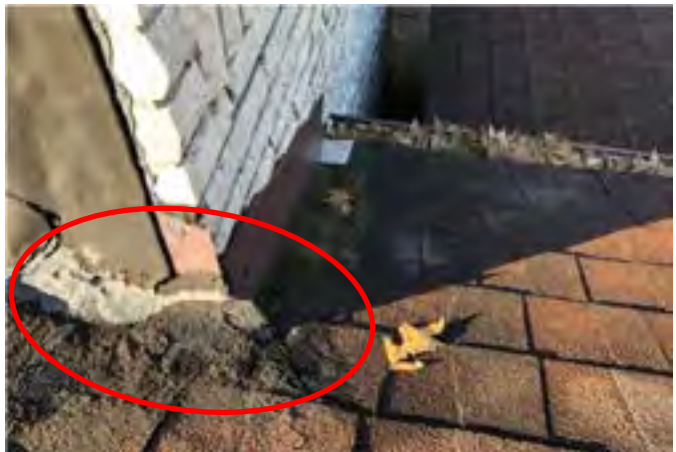
Steep slope roof-to-wall and low-slope to steep slope roof transition with several applications of roof mastic. This is most likely a source for moisture infiltration.
