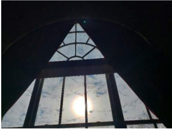
Photo 9 -Broken Window Frame
