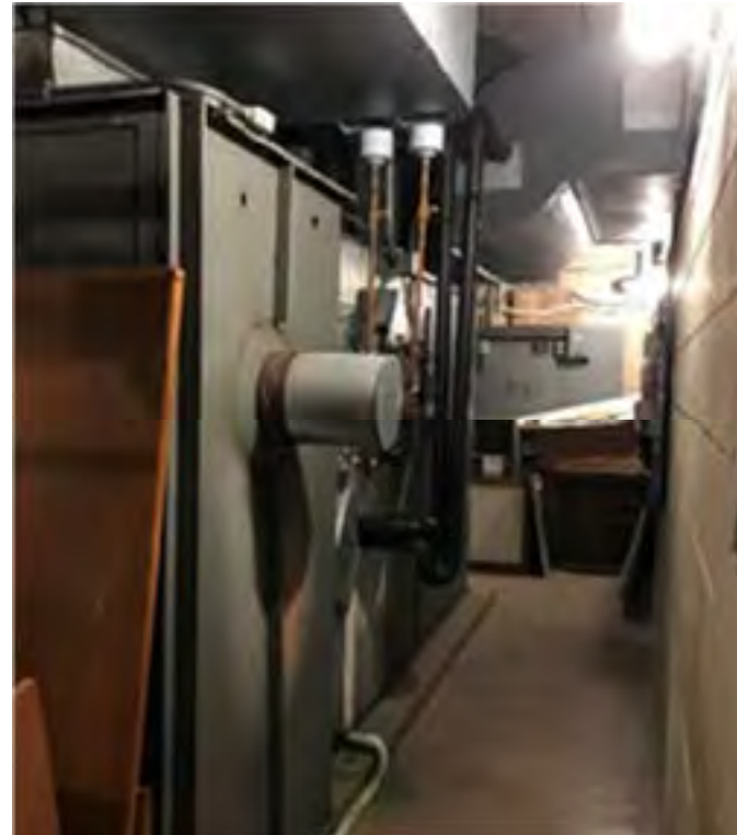
1961 Air Handling Unit
