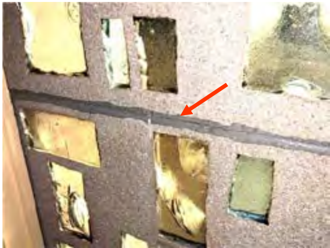
Failed sealant on the interior of the Art Deco panels.
