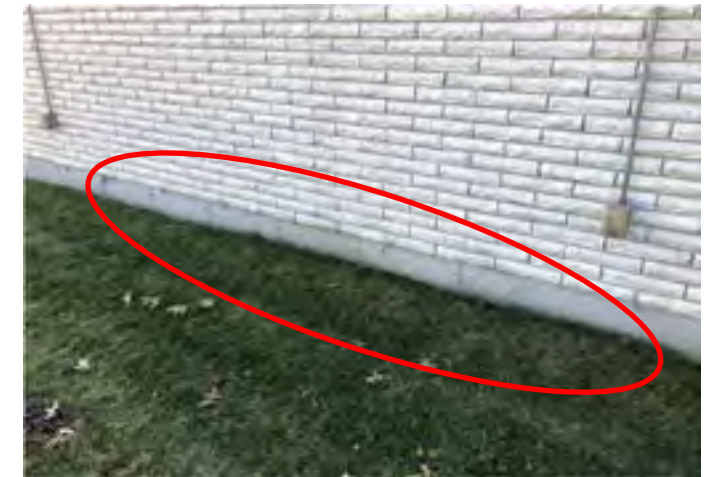
Weeps observed at base of wall.
