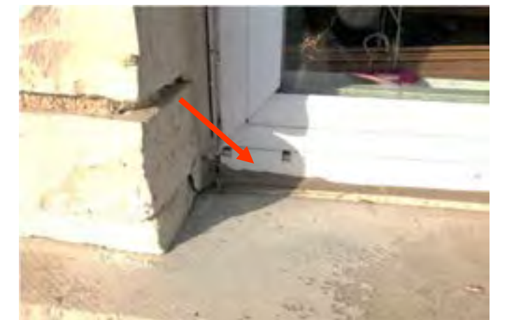
Failed sealant was observed at several windows on the Parish Center.
