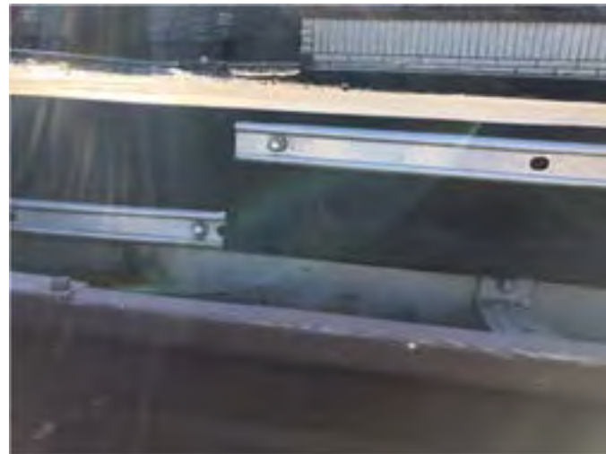
Poor termination bar installation at low slope, fully-adhered, EPDM roof area.
