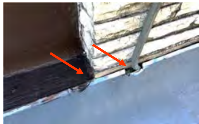
There is no watertight seal between the exterior and the sheet metal flashing cover to prevent water from infiltrating.
