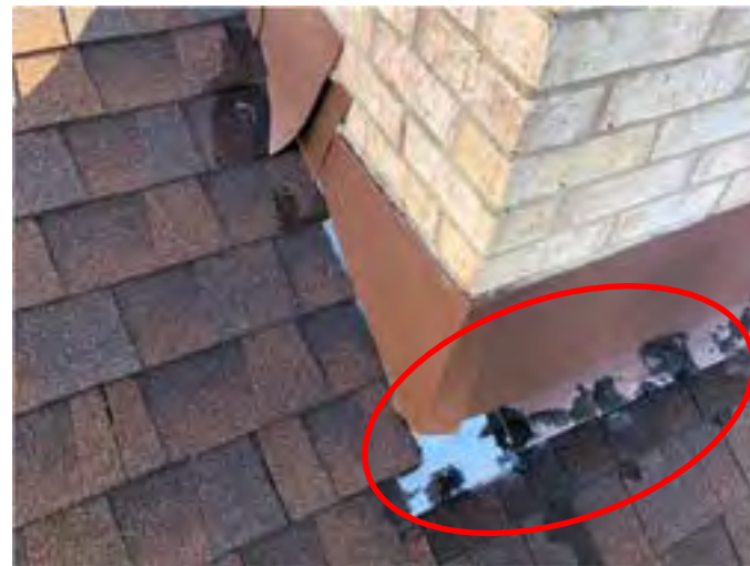
Multiple applications of roof mastic observed at skirt flashing on down slope of chimney flashing on Narthex roof.
