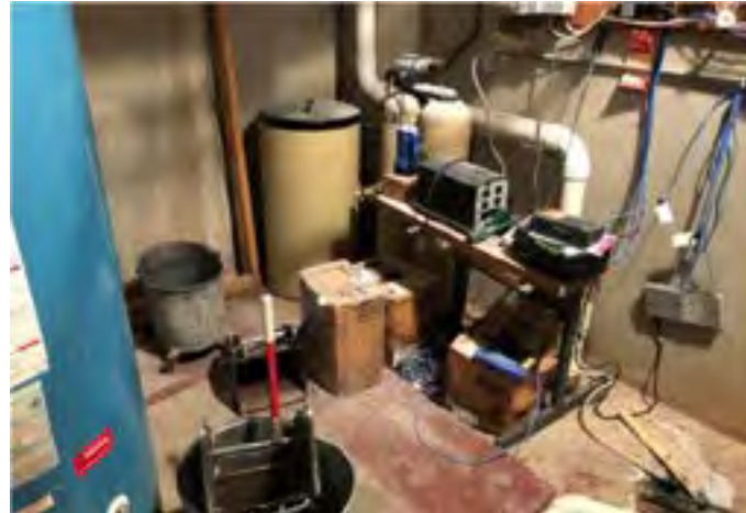
Water softener system. No current leaks in foundation observed.
