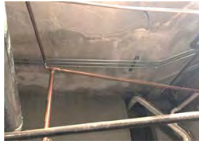
Ceiling condition along west wall of mechanical room. Previous moisture staining was observed but no active leaks at the time of this assessment.
