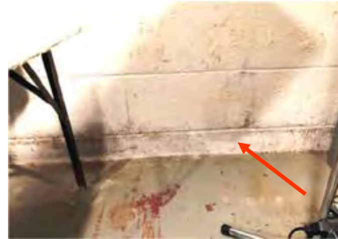
Efflorescence and peeled paint at the base of the wall
