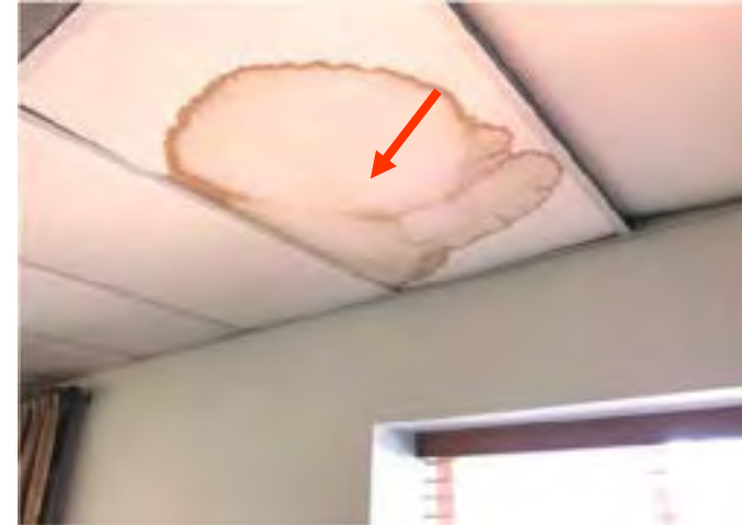
Moisture stain along west elevation wall.
