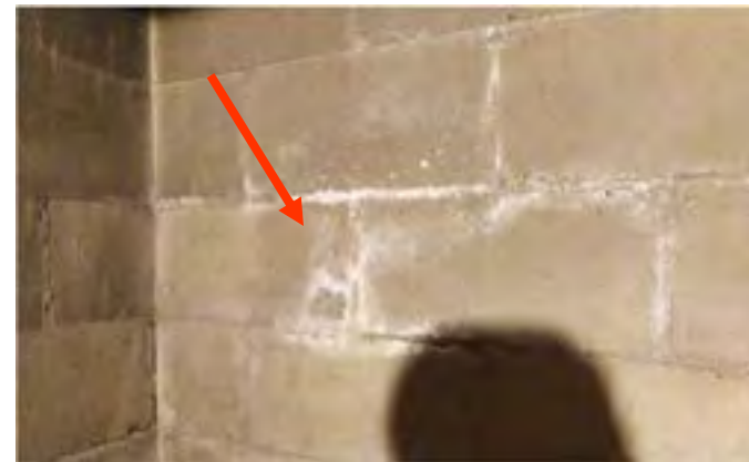
View of efflorescence on the interior surface of the basement living quarters.
