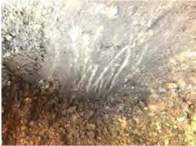
No water/dampproofing observed on the Church foundation.
