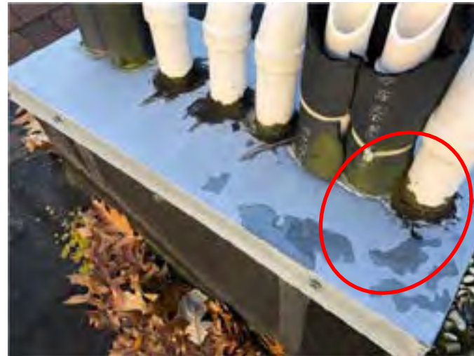
Failed sealant observed at multiple pipe flashing penetration curb.
