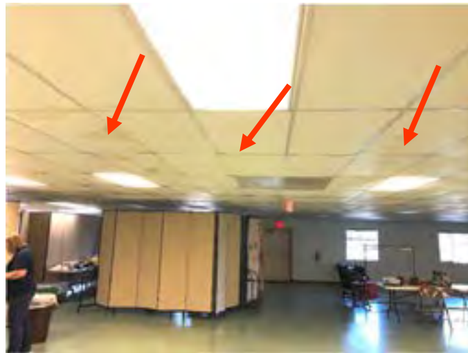
Drop ceiling inside the Parish Center. Note: Moisture stains, and no staining in between.
