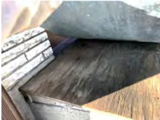
Plywood is damp and moisture leaks under the metal cover.
