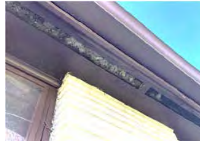
More debris observed in soffit vents at the chapel.
