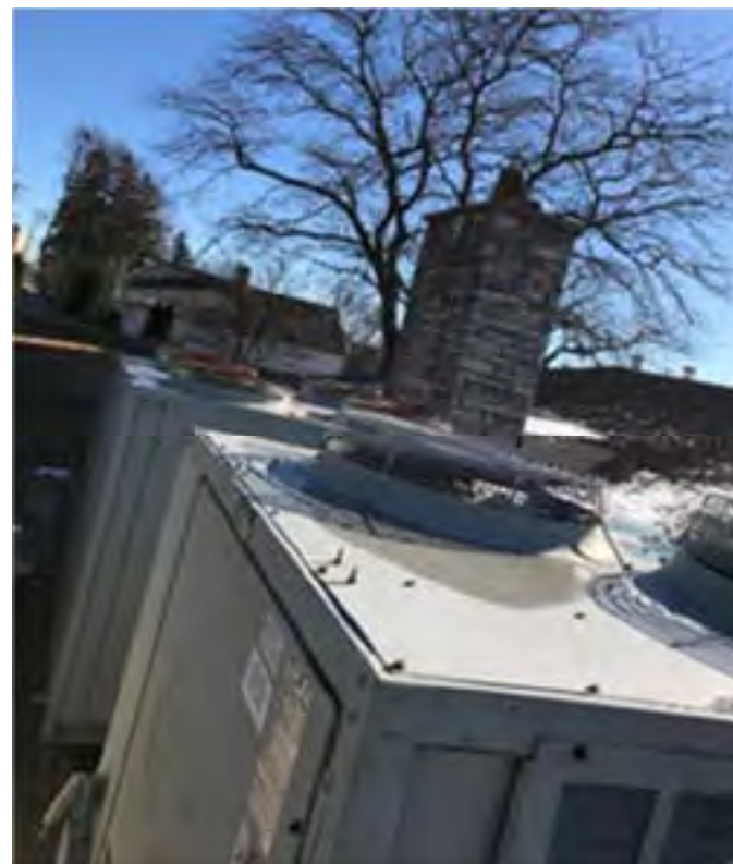
2001 Air Cooled Condensers
