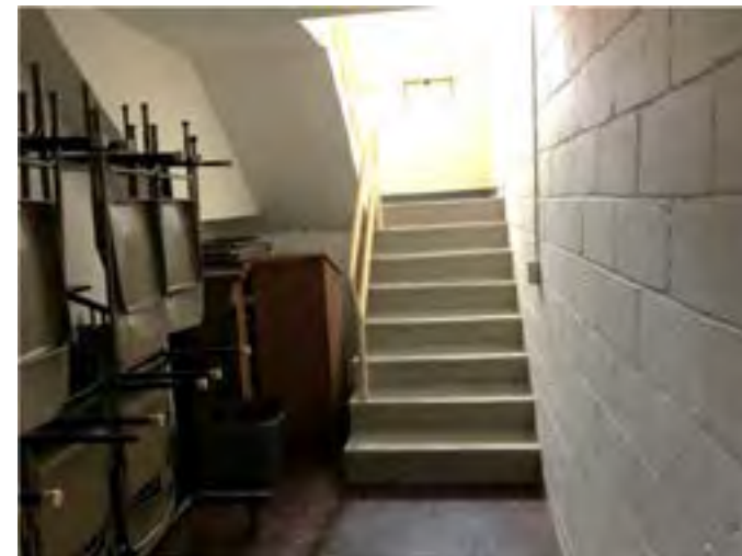
Stairwell leading up to Church. No active leaks observed.
