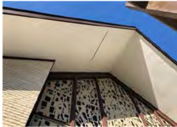
Soffit panel is loose near the peak of the Church entrance.
