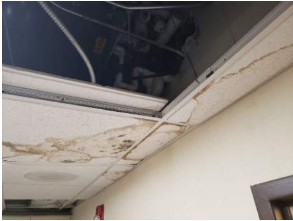
Photo 12- Stained Ceiling Tile
