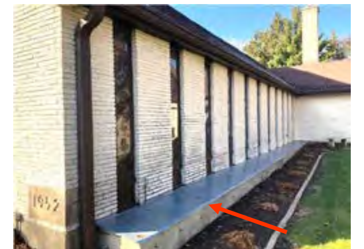
Sheet metal and plywood light well cover on north side of Church is not adequately weatherproofed.
