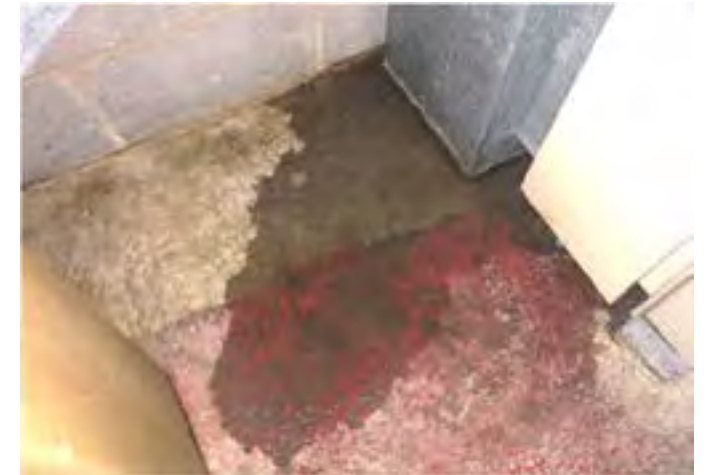
Visible moisture observed at the base of the east wall of the mechanical room.
