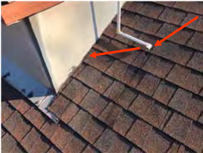
View of deflection in roof decking at HVAC condensate drain.
