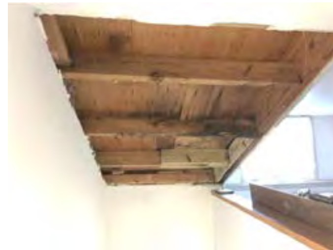
Drywall ceiling removed at chapel upstairs storage room. Note: Moisture stains observed at roof-to-wall transition suggests a step flashing issue.
