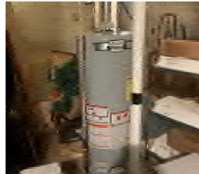
Gas Water Heater
