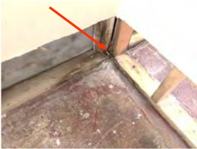
Noticeable moisture damage was observed.
