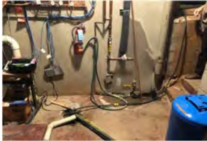
View of mechanical room below the Narthex. Visible water is from water piping and condensation.
