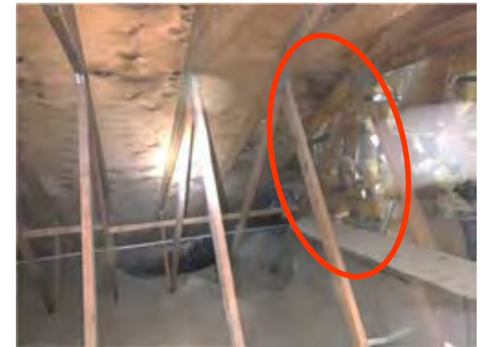
Evidence of moisture staining next to HVAC unit ductwork.
