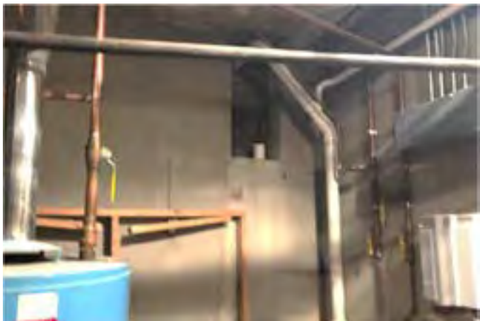
Opening in foundation wall along west side of mechanical room, no active leaks were observed.
