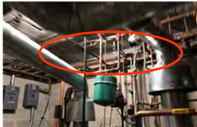
View of mechanical room to the north that houses the hydronic heating for the Parish Center.
