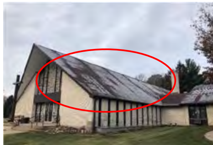
Hot spot locations observed on north slope of the Church
