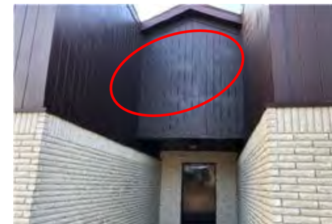
Interior alcove at north end of the Parish Center. Several touch-up applications of paint were observed
