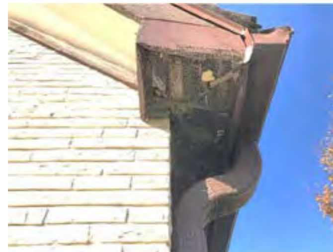
Soffits on the chapel appear to be blocked with debris from within the rafter spaces.
