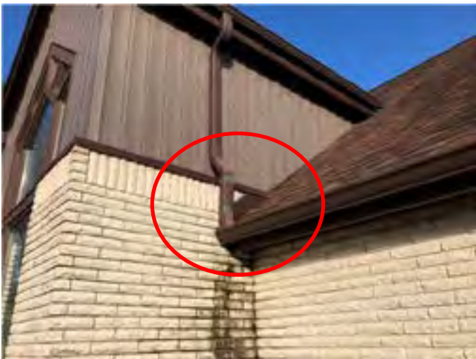
Roof-to-wall transition that lacks a kick-out flashing to divert water into the gutter
