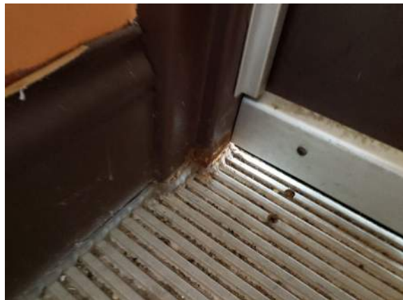
Photo 11 - Door Frame Corroding
