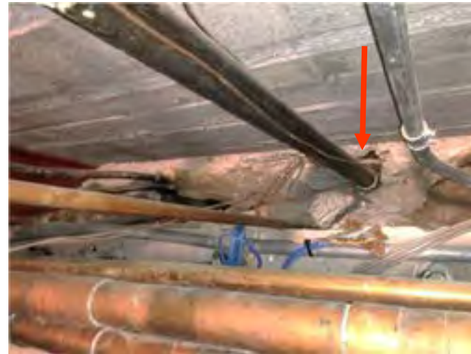
Hydronic piping going into wall/floor of the Parish Center above.
