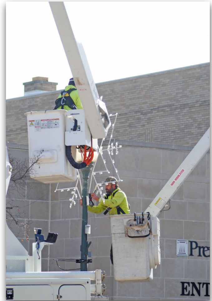
MEMBERS OF THE DEPARTMENT OF PUBLIC WORKS PUT UP CHRISTMAS LIGHTS ON MAIN STREET.
