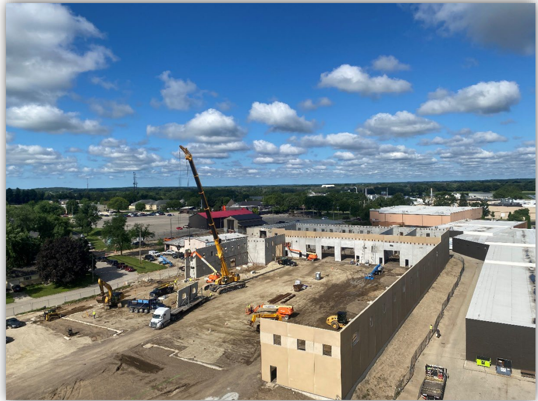
THE DEPARTMENT OF PUBLIC WORKS AND PARKS FACILITY CONSTRUCTION IS SEEN EARLIER THIS SUMMER.
