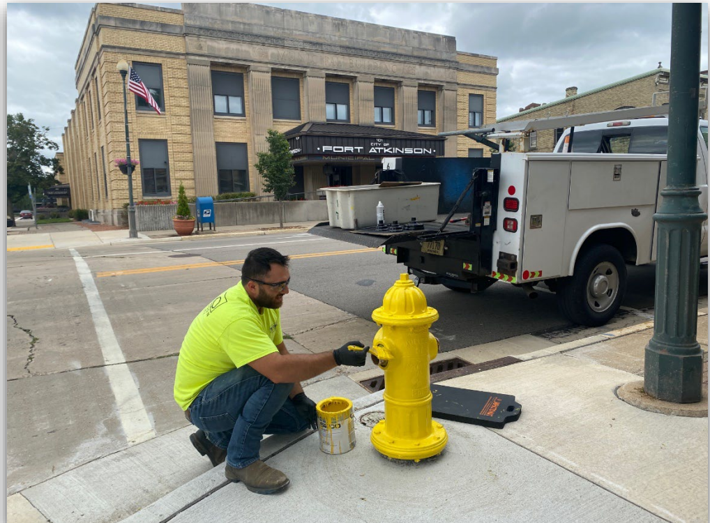
KORADO LUFTA IS SEEN IN AUGUST PAINTING A FIRE HYDRANT ON MAIN STREET.
