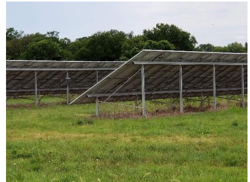
Example of a Solar Conversion System, Ground-mounted
