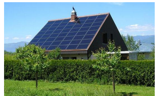
Example of a Solar Conversion System, Structure-mounted
