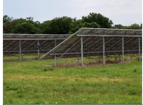
Example of a Solar Conversion System, Ground-mounted
