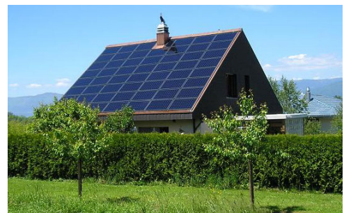
Example of a Solar Conversion System, Structure-mounted
