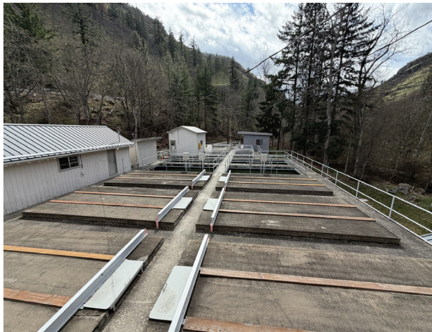
Wicks Water Treatment Plant built in 1949
