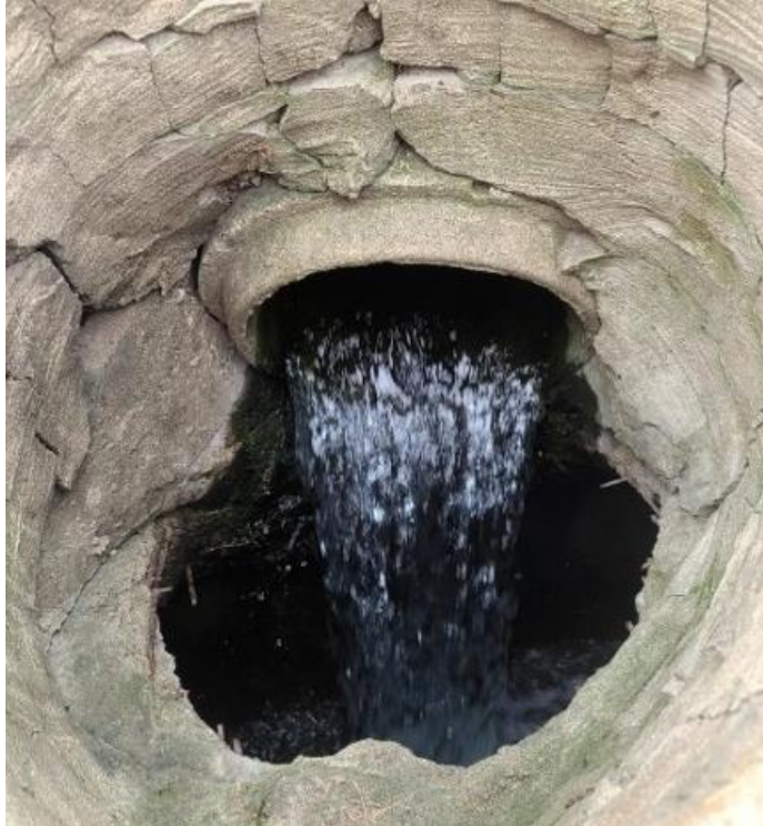
Geothermal system at Franklin Middle School – Valve left open leading to constant discharge
