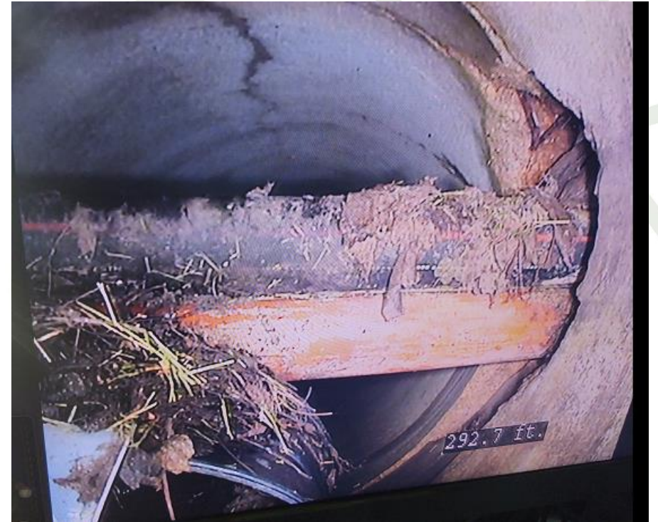
Utility cross-bores limit capacity of sewers and trap debris that causes blockages
