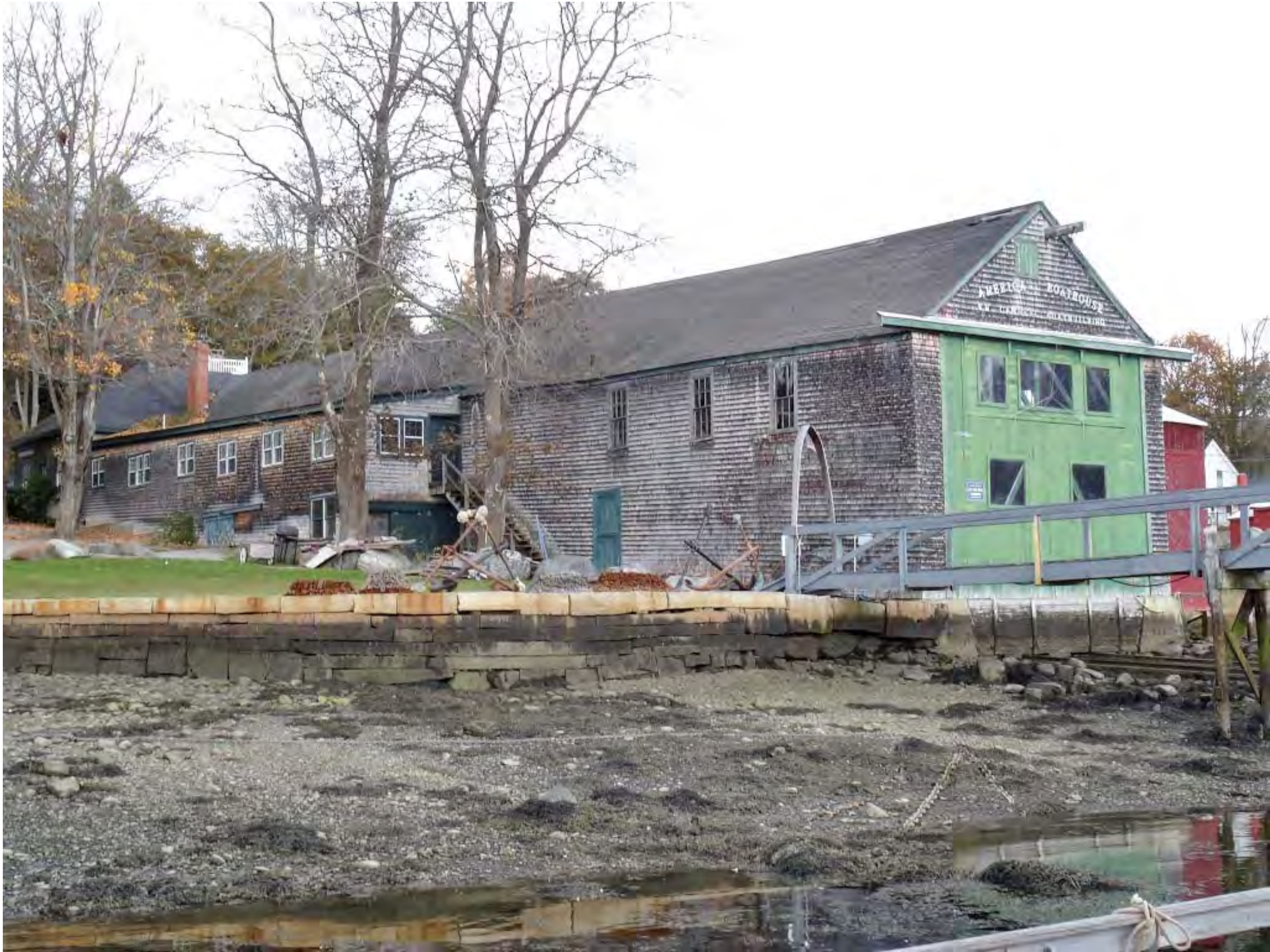
EXTERIOR EXISTING CONDITIONS IMAGES American Boat House 17 Atlantic Avenue, Camden
